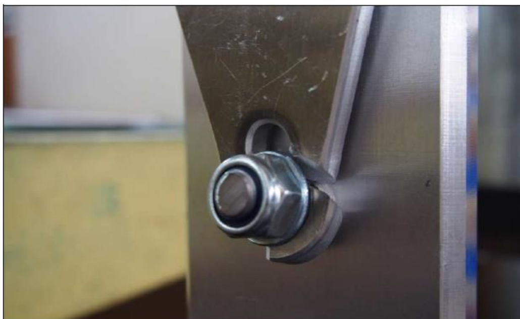
Pic. 4. Destroyed bolts connection in the hub bar
